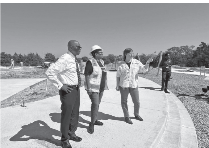
Dallas City Council member Tennell Atkins, Rep. Toni Rose, and Trust for Public Land's Texas State Director Molly Morgan survey the ongoing construction of the Judge Charles R. Rose Community Park
